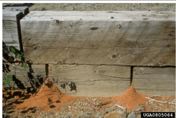
Fig. 1. Sawdust from carpenter ants near a retaining wall timber. (Edward H. Holsten, USDA www.bugwood.org )
